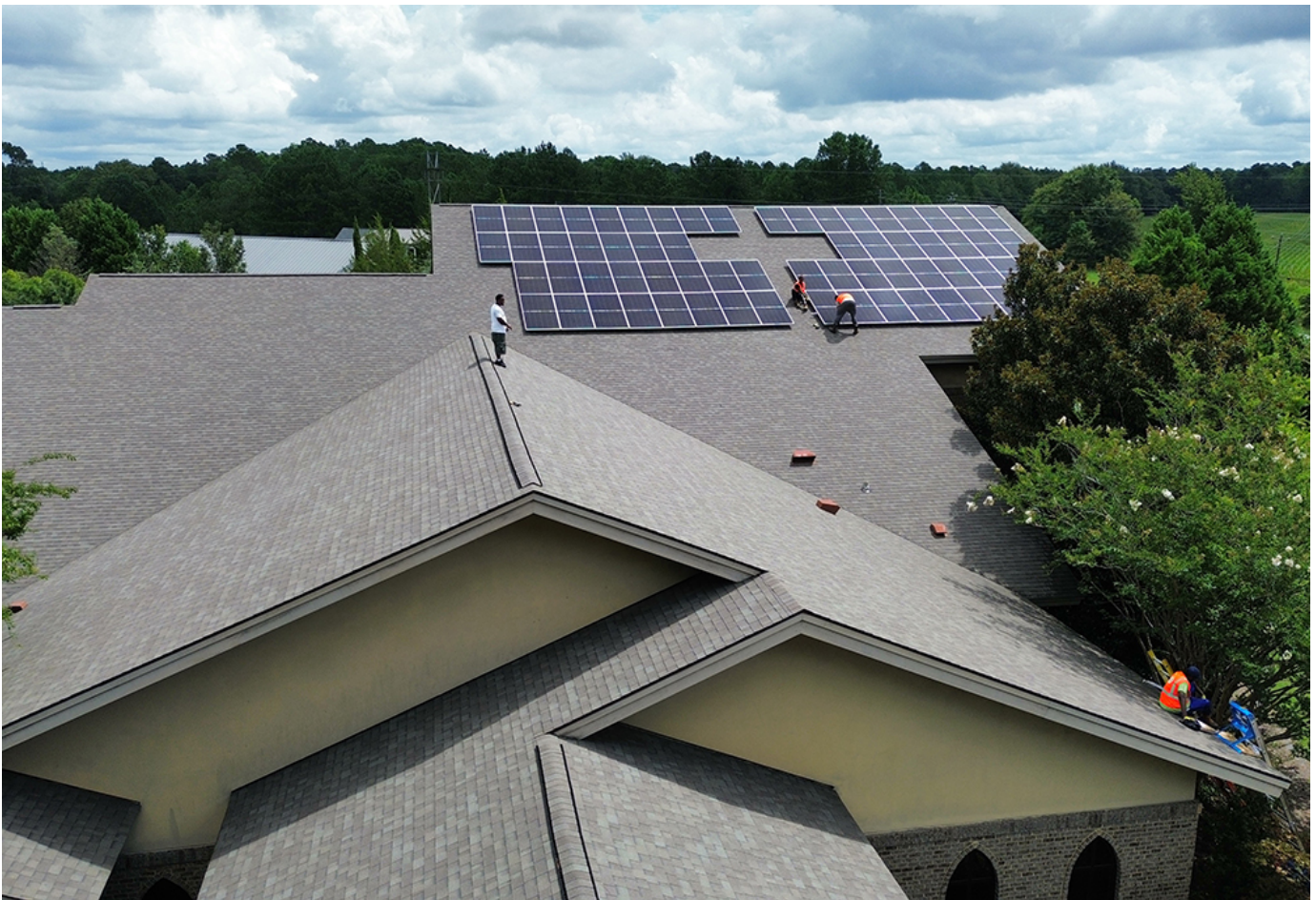
A solar installation is pictured at Trinity Episcopal Church in Statesboro, Georgia, on July 25, 2024. (Courtesy of Sunpath Solar and Georgia Interfaith Power and Light)
