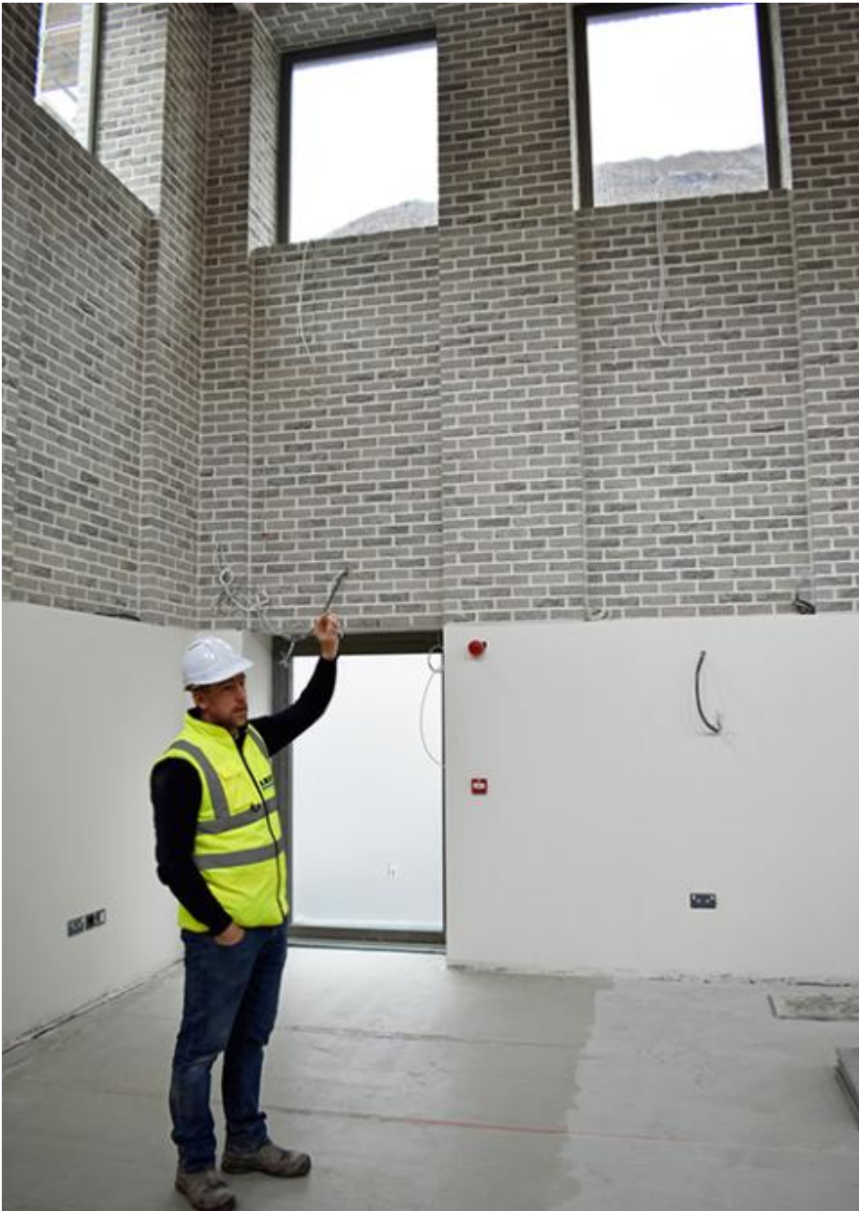
David Connor, Carey Building Contractor's site manager on the Kylemore monastery project, explains the intricate brickwork around the high windows created for the multipurpose room. (Julie A. Ferraro)
