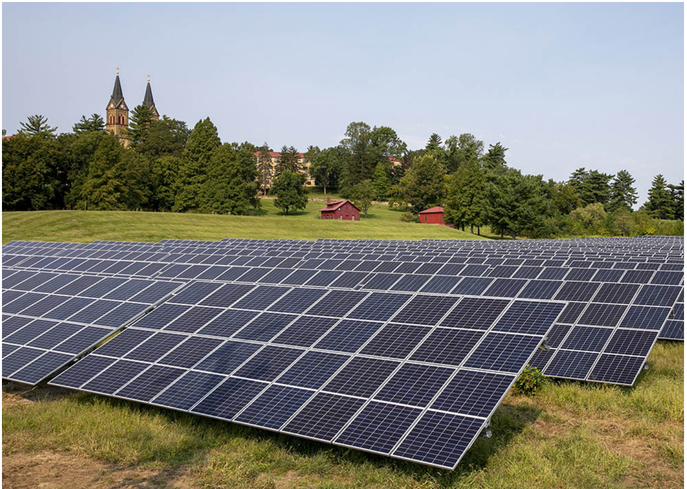
Solar panels are seen on the campus of St. Meinrad Archabbey and its seminary in Spencer County, Indiana, Sept. 11, 2021. (CNS/Courtesy of St. Meinrad Archabbey via The Criterion)
