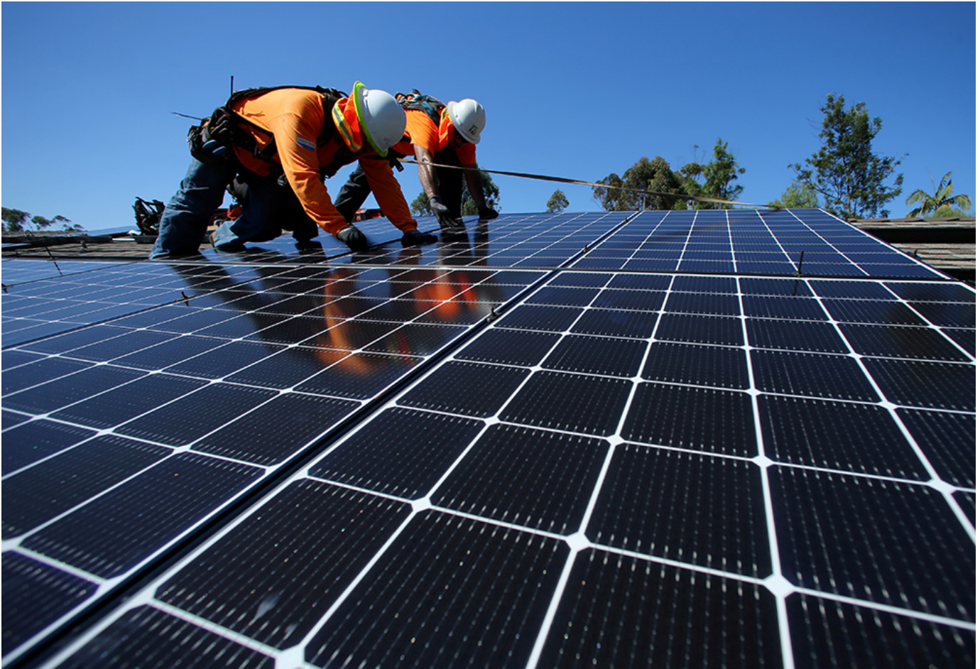
Solar installers are seen on a residential home Oct. 14, 2016, in Scripps Ranch, California. (CNS/Reuters/Mike Blake)
