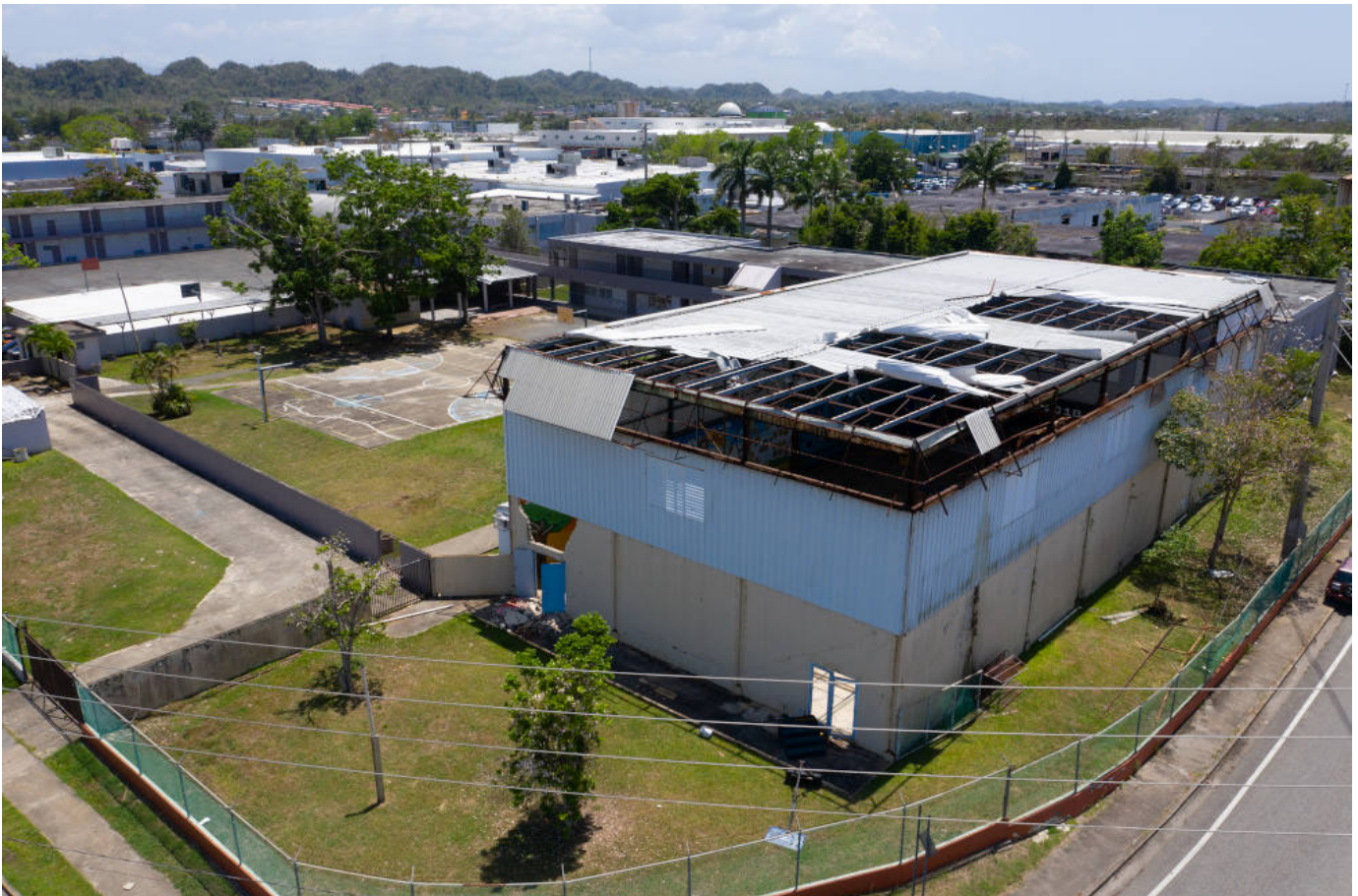
The damaged gymnasium of Colegio Nuestra Señora del Rosario in Vega Baja, Puerto Rico, in 2019. The school was damaged in 2017 by Hurricane Maria. (RNS Photo/courtesy of Catholic Extension.)
