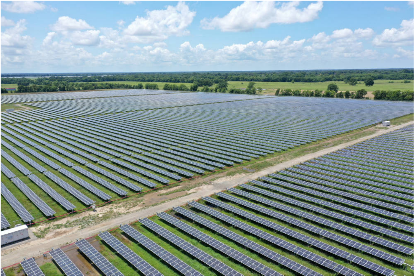
Solar panels are seen in Deport, Texas, July 15, 2021. (CNS photo/Drone Base, Reuters)
