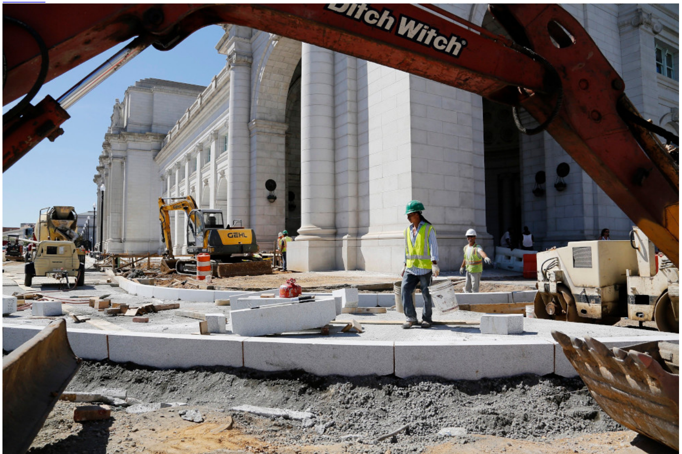
Construction workers rebuild the driveway in front of Union Station in Washington July 25, 2012. (CNS photo/Reuters/Jonathan Ernst)
