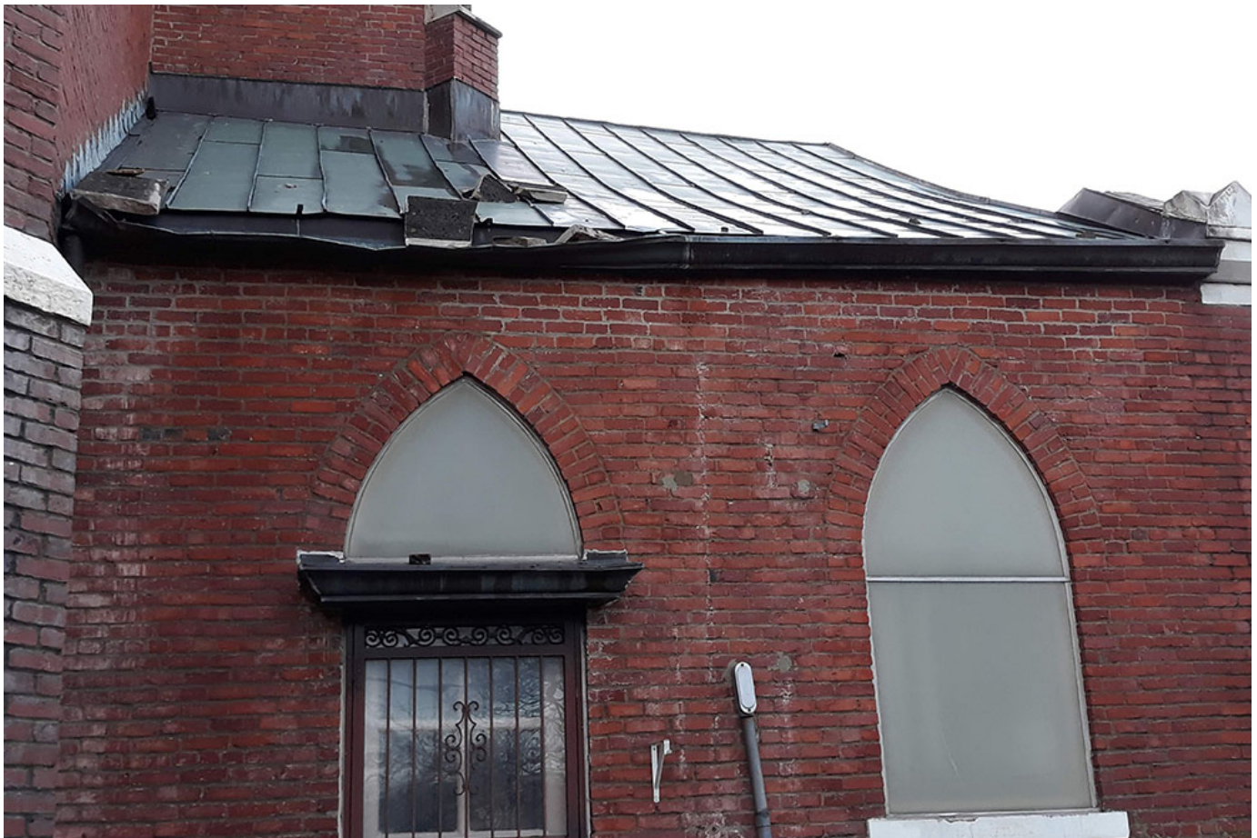
Sacristy roof damage at Assumption Church in Nashville, caused by the March 3 tornado (Mark Cassman)
